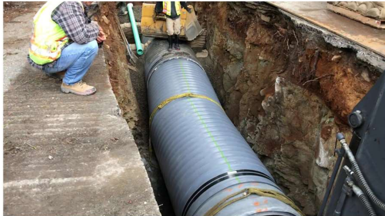
SaniTite HP pipe made it possible to have five-degree bends prefabricated at the ADS plant to accommodate the terrain and to follow the road. Credit: ADS
