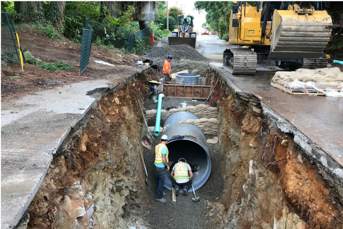
The new pipe system will enable storm level flows to be managed within the Five Creeks area of West Vancouver and will reduce the impact of intense storms in Westmount and West Bay. Credit: ADS
