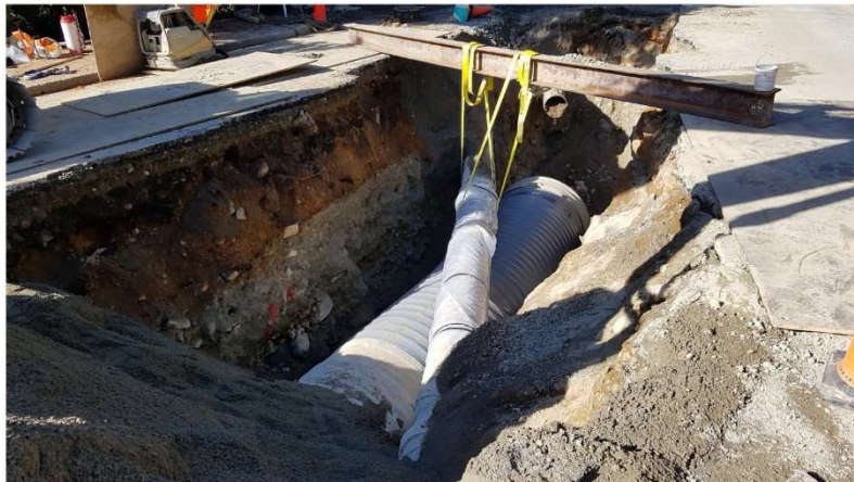
It was possible for the contractor to slip the large diameter stormwater pipe under existing utilities. Credit: InterCAD
